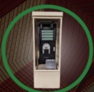
288 Fiber Cabinet with Splitters
