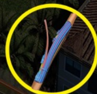
Duct Access Point
