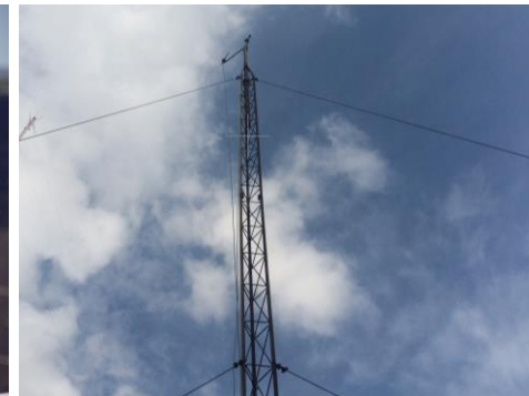
Wind Mast – traditional wind monitoring
