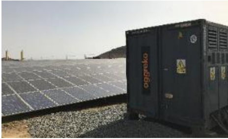
Solar Power Pack
